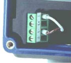
View of terminal block with front cover removed
